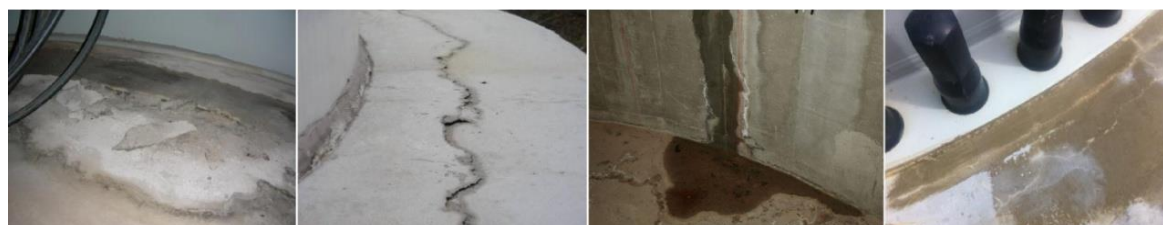
Spalling inside Spalling outside Water intrusion Circumferential cracks
