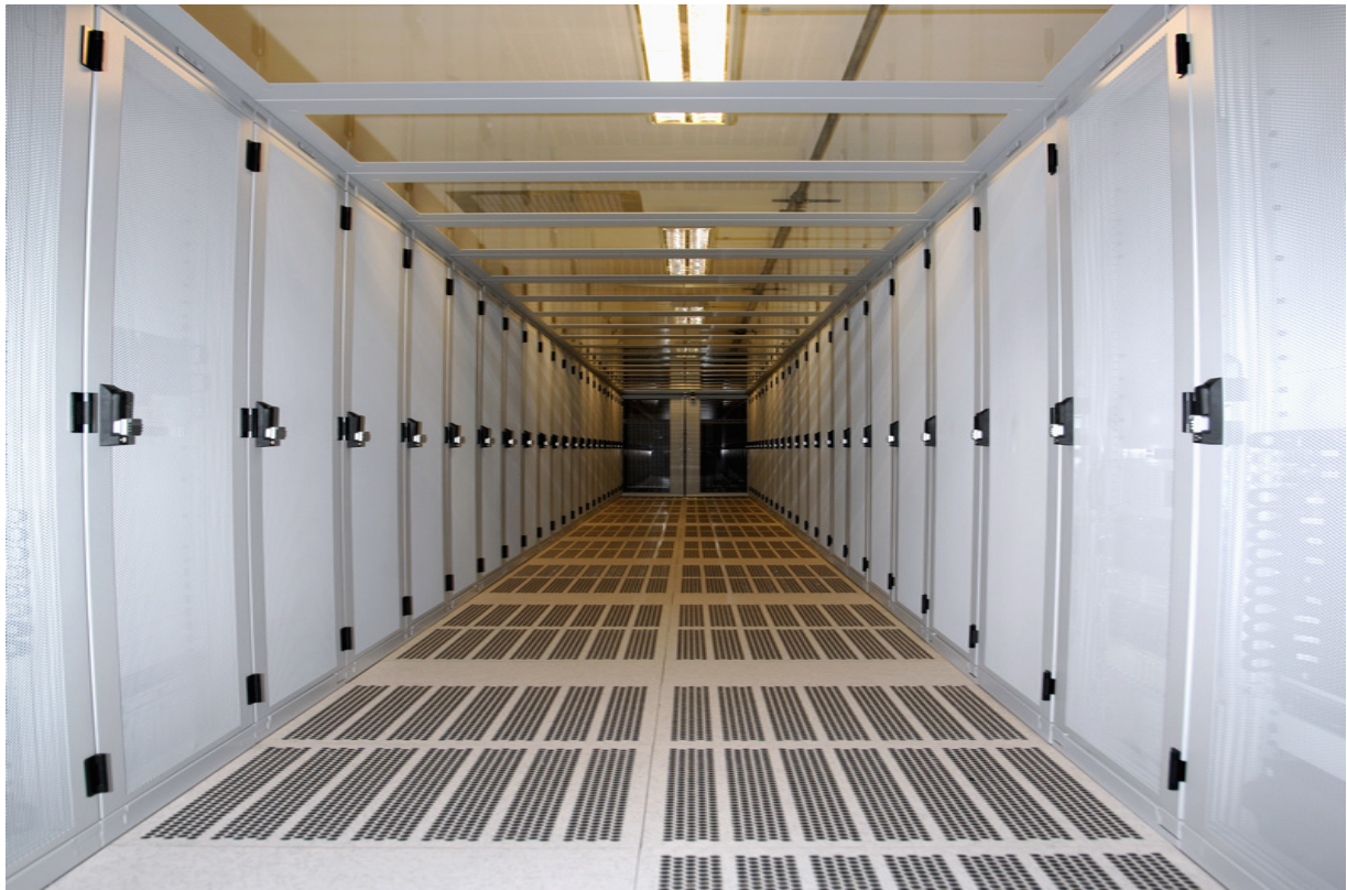
Figure 4: picture of the Unisys computer centre: large numbers of servers needed
